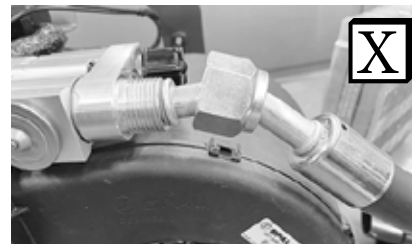
Improperly Seated O-ring Land
