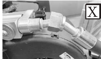
Improperly Seated O-ring Land
