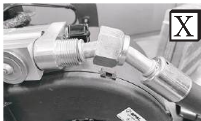
Improperly Seated O-ring Land
