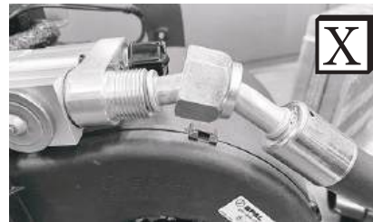
Improperly Seated O-ring Land
