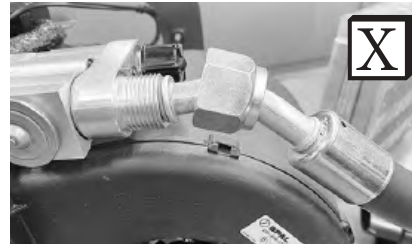
Improperly Seated O-ring Land
