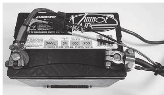
Completed Installation Shown
