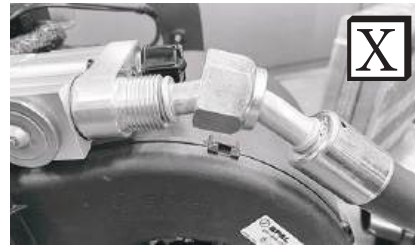
Improperly Seated O-ring Land
