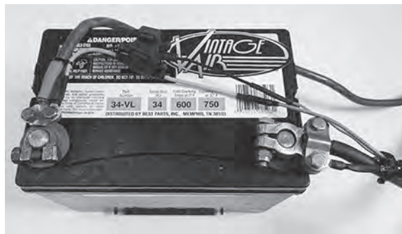
Completed Installation Shown
