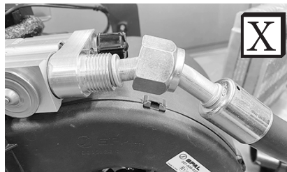
Improperly Seated O-ring Land
