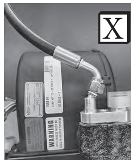
Improperly Seated O-ring Land
