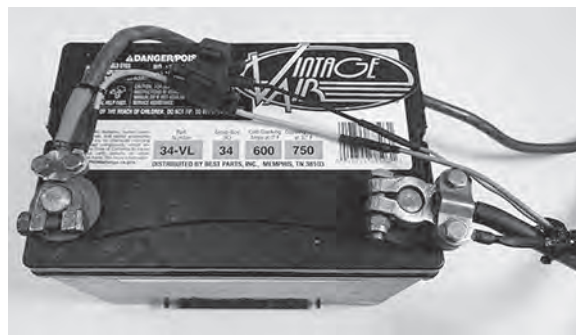
Completed Installation Shown
