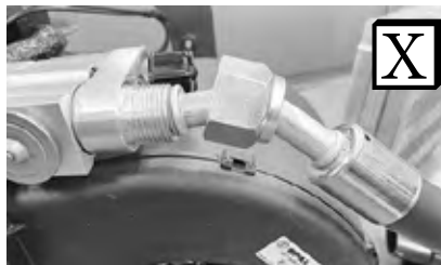
Improperly Seated O-ring Land
