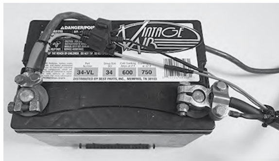
Completed Installation Shown
