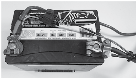
Completed Installation Shown
