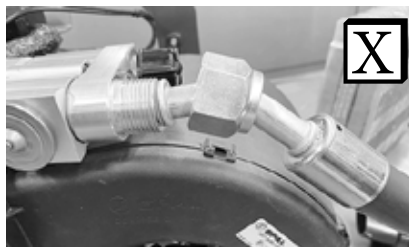
Improperly Seated O-ring Land
