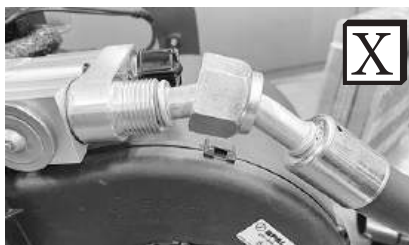
Improperly Seated O-ring Land
