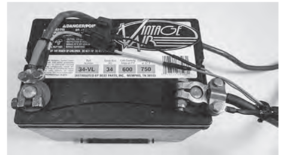
Completed Installation Shown
