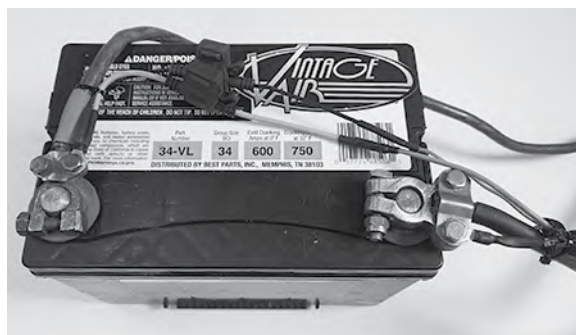
Completed Installation Shown
