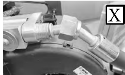
Improperly Seated O-ring Land
