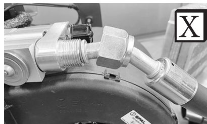
Improperly Seated O-ring Land
